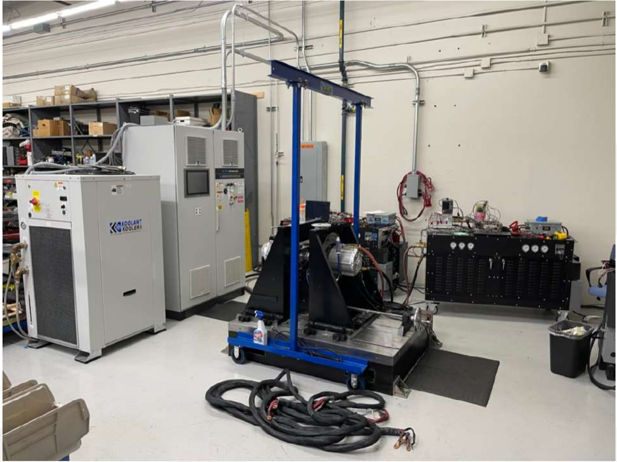
Pre-Switch lab: 250kW 3 Phase AC/DC PSU & Dynamometer
